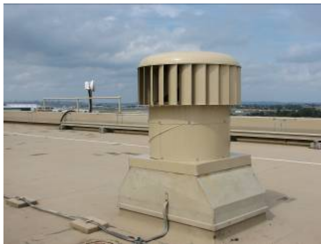
Figure 6: ecopower installation on ventilation shaft on Mercure Hotel Sydney Airport.
