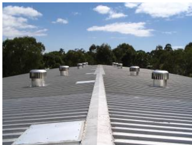
Figure 7: ecopower installation in Alexandra Hills State High School QLD.
